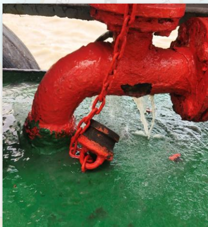
Wasted fire line on deck
