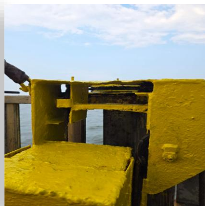
Pilot combination ladder sheave housing thinned down
