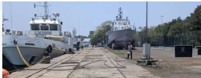
1600 KVA Ship to Shore power supply
