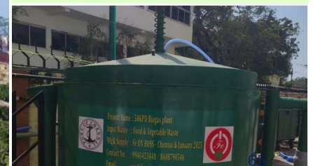
50 KPD Biogas Plant
