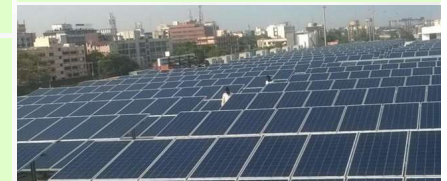
500 KW Roof top Solar plant
